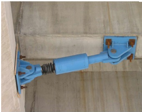
Typical anchoring configuration of a fluid viscous device (photo taken during the installation).
